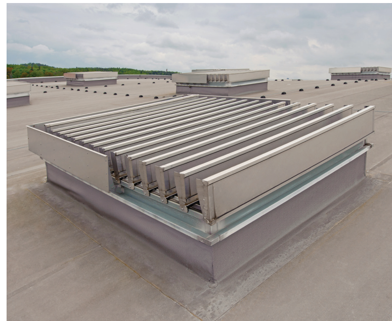
Fig. 36 - mcr LAM louvered vent, roof mounted
