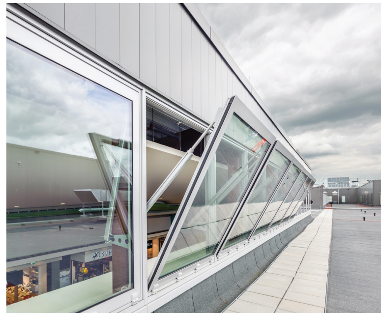
Fig. 32 - mcr OSO THERM smoke exhaust windows open
