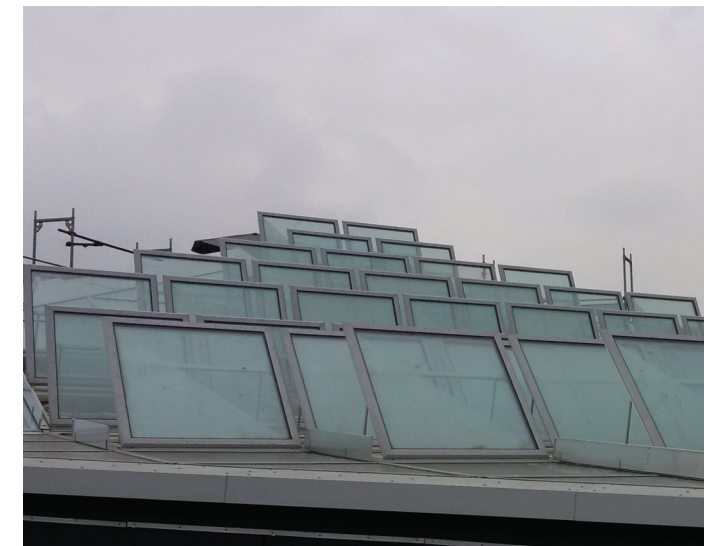
Fig. 35 - mcr OSO THERM smoke exhaust windows, open
